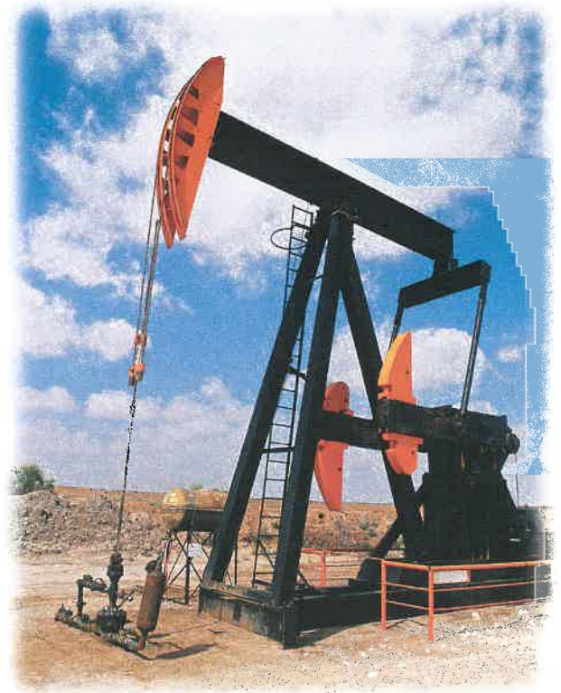
Pumpjack with natural gas engine
